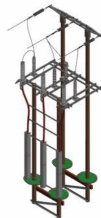
Typical Trident cable terminal pole
